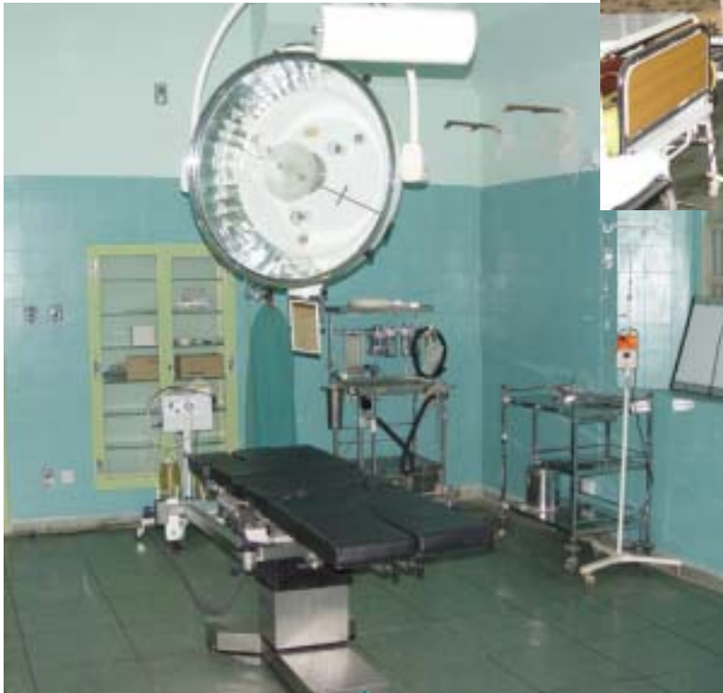
Operating Room number one (of 2) at K-1 Hospital.
